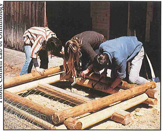
Constructing a loon nest platform can be a good project for a lake association.
